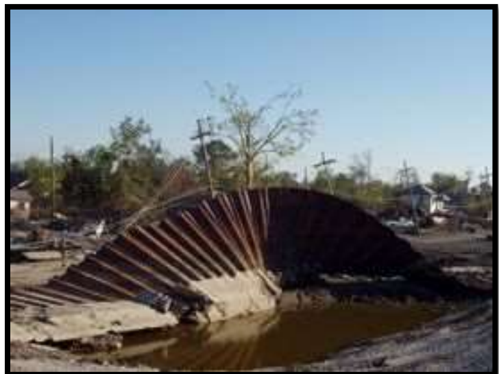
Failed Sea Wall in the 9th Ward of New Orleans. Photo National Park Service.
