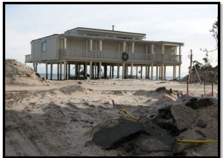
Residential home being raised to adhere to Base Flood Elevations. Photo courtesy of FEMA
